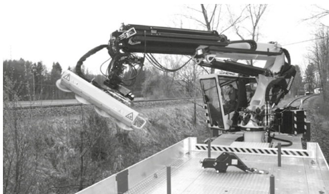
KM 931-500 at a fix crane on a railway wagon (here with a branch saw)
